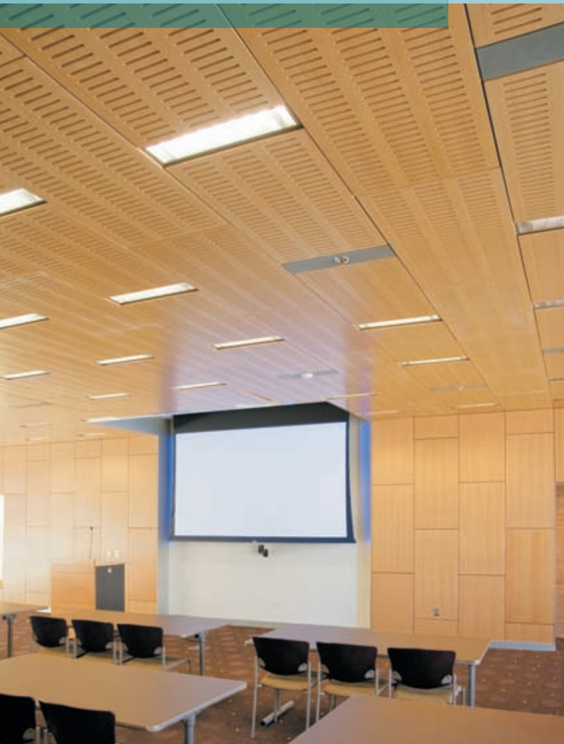
WoodWorks Wall 2' x 4' panels on Z-clips and Ceiling 2' x 4' panels with custom perforation (running parallel to the short side of the panel) in custom Vertical Grain Douglas Fir
